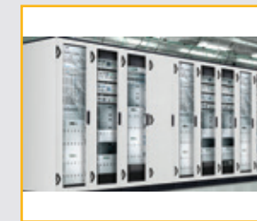
Signalling & Passenger information systems
